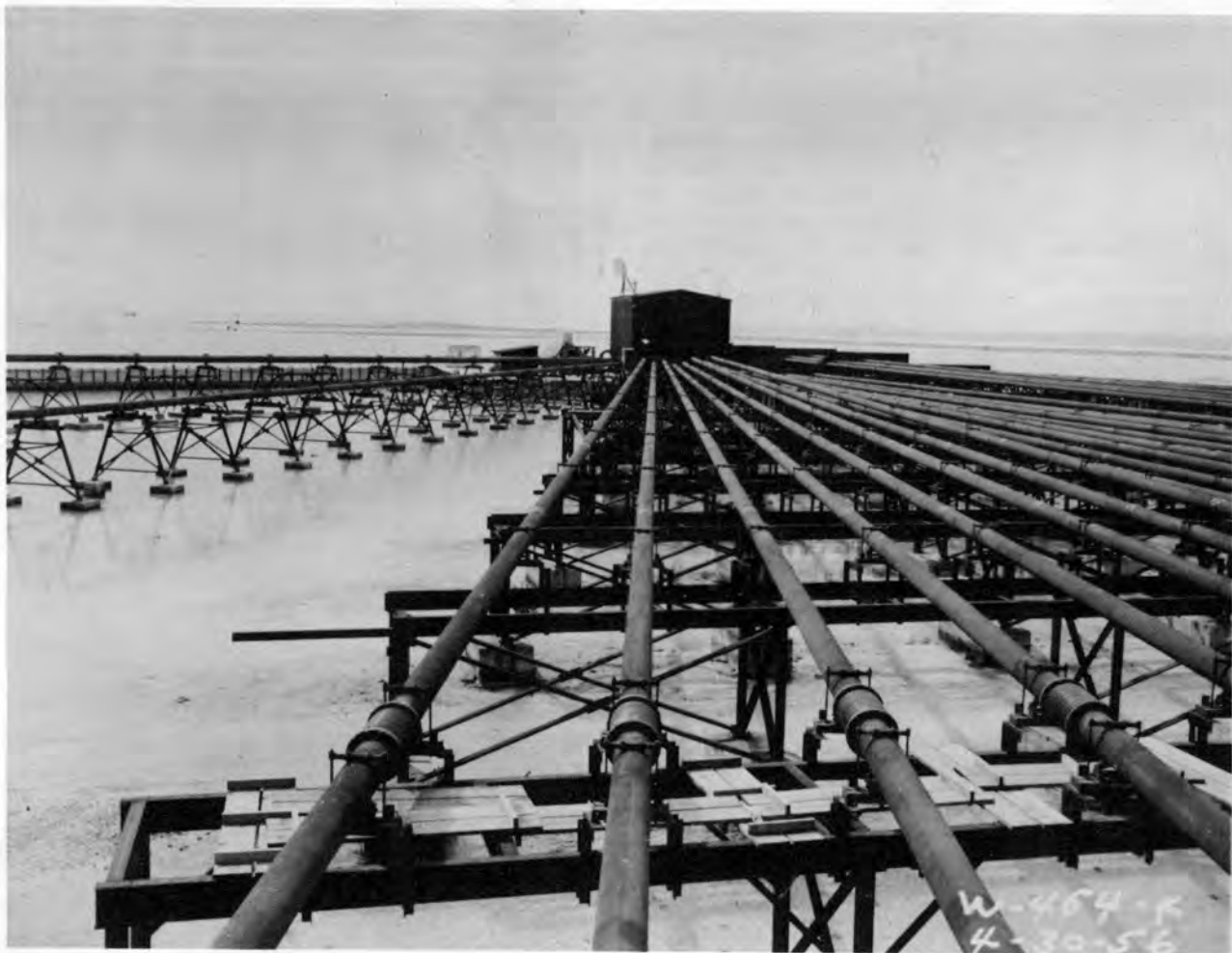
Figure 2-40. Pipe Arrays Leading to Station 24
